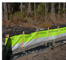
Silt Saver Silt Fence Outlet
