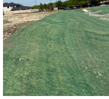
Excelsior ECB's Temporary
