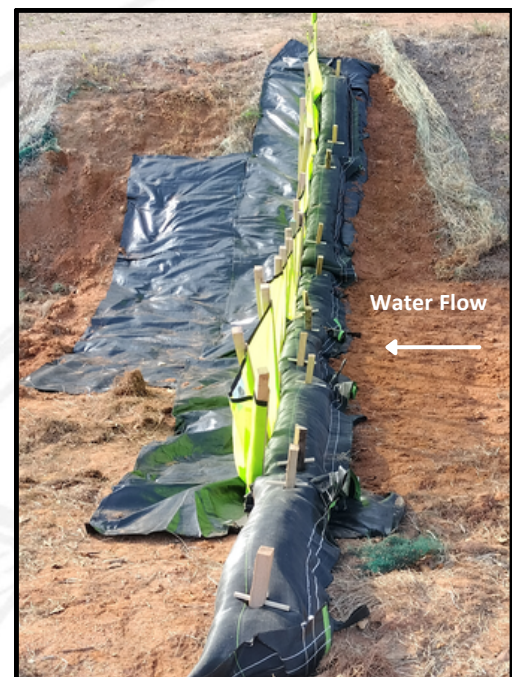
Rear scour guard
